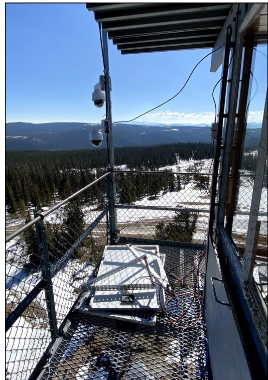
Figure 10— Storm damaged solar panels at the Deadman Lookout site
