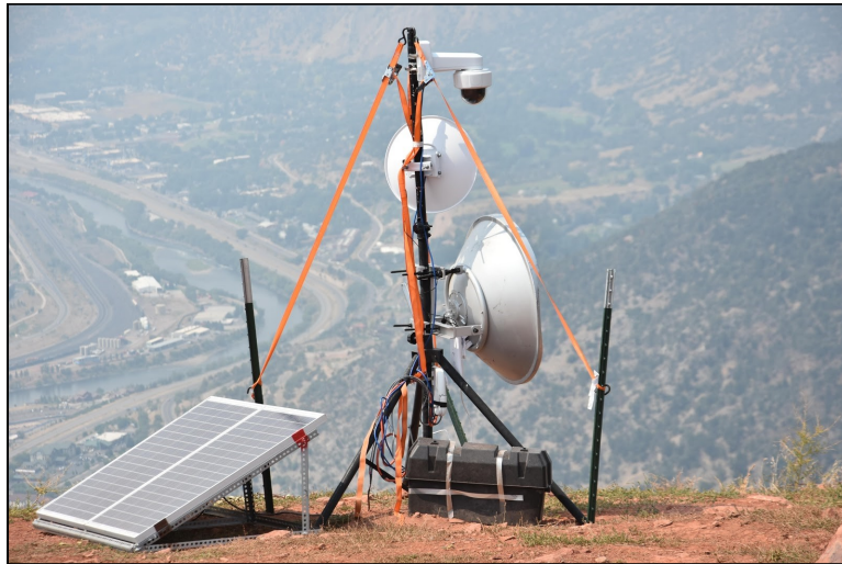
Figure 4— Equipment installed at Lookout Mountain
