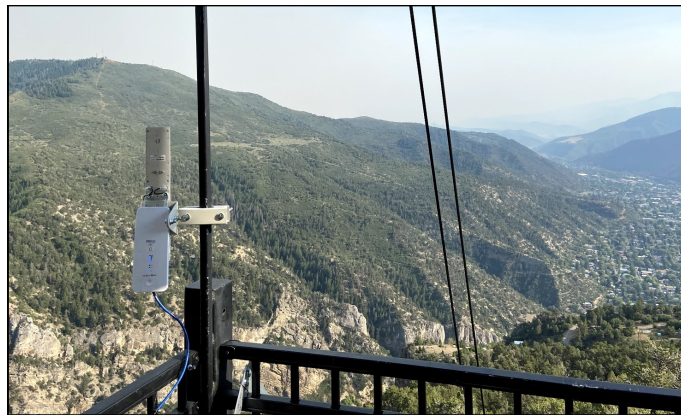
Figure 3— Repeater radio at Glenwood Adventure Park
