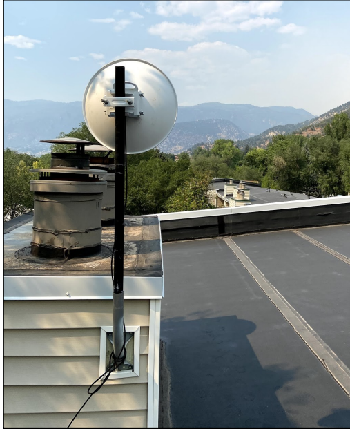
Figure 2— PowerBeam installed at home of CoE staff member in Glenwood Springs
